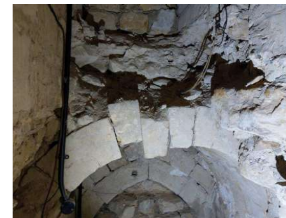
View from Tower passage showing Norman arch with displaced voussoirs.
