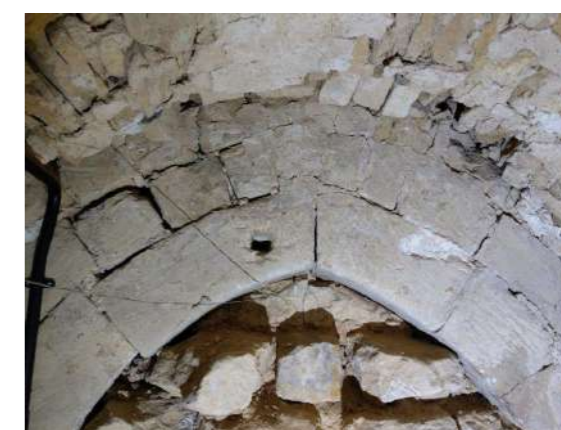
View from Tower passage showing pointed inner arches and blocked up entrance
