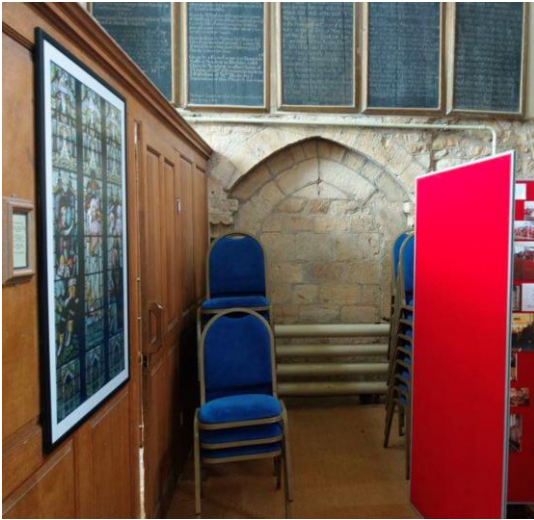
The blocked-off access into the tower. - Small pointed arch within a larger pointed arch which replaced an original Norman rounded arch!
