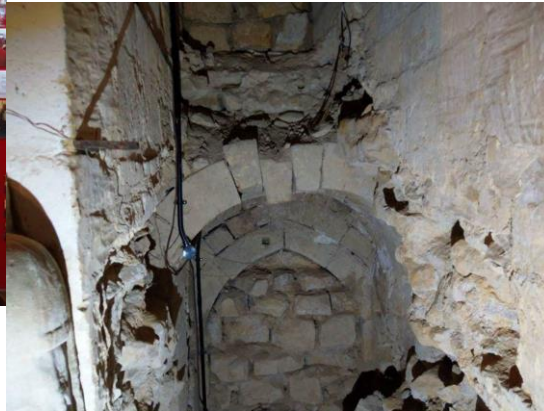
From the tower side, it is a mess and needs work to stabilise it.
